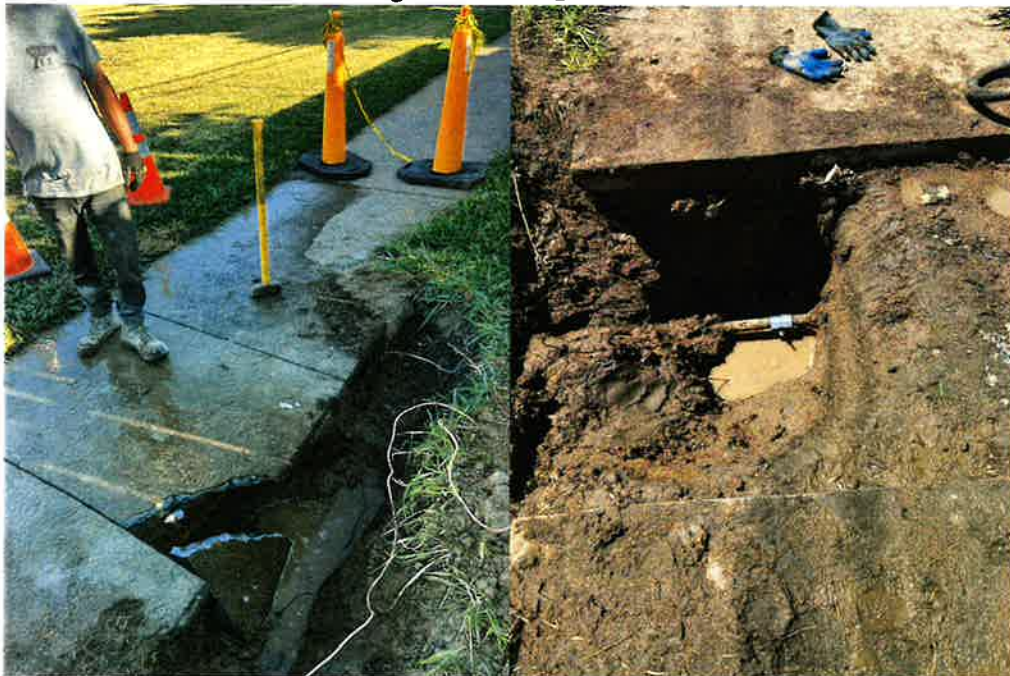
Irrigation Leak @ Strizek
