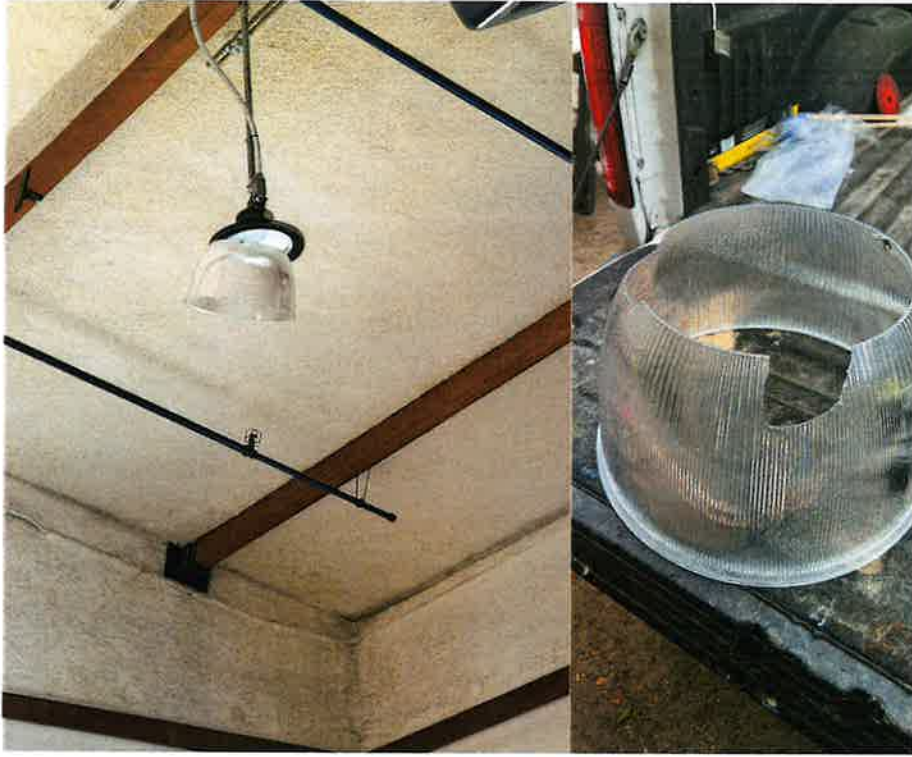
Broken Light @ Capehart
