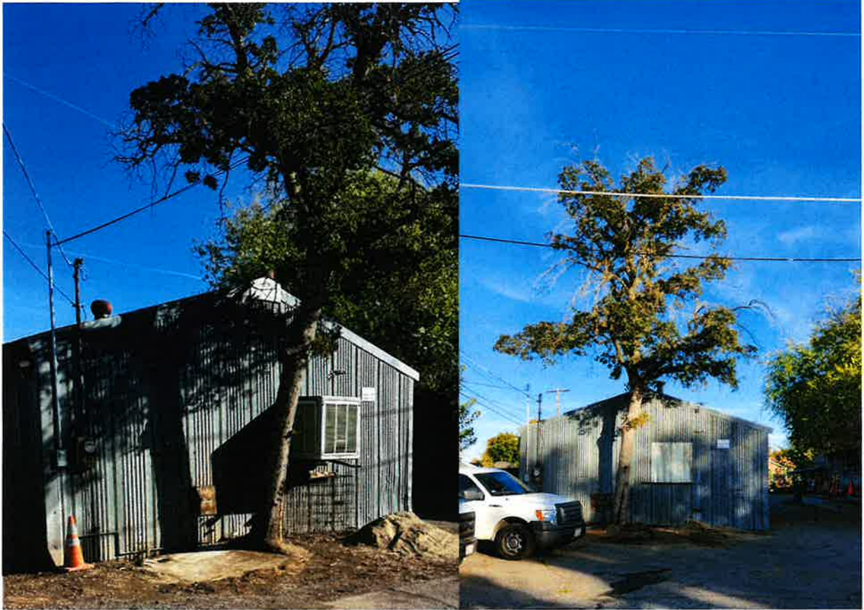
Dilapidated Shed (cont.)
