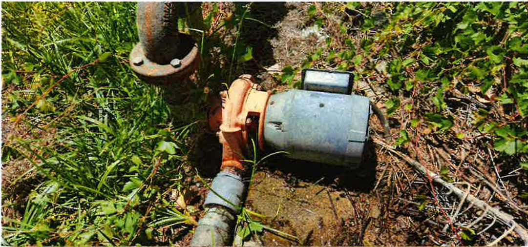
Capehart Booster Pump
